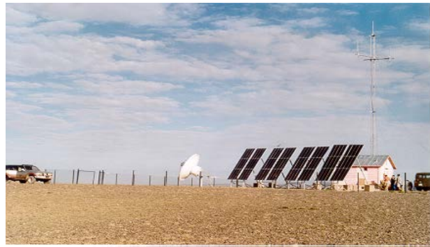
Figure 19. Photovoltaic Power Generation System in Rural Area
