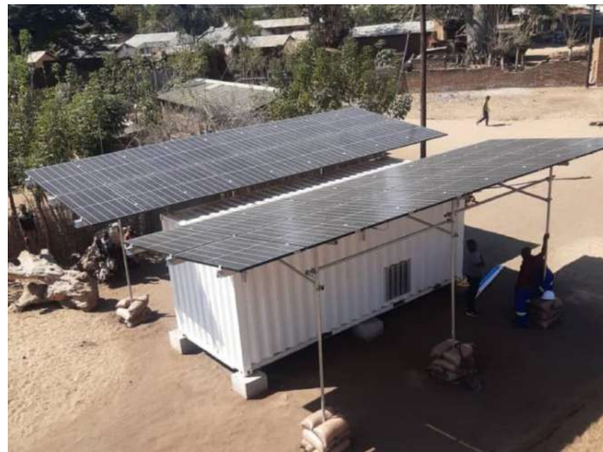
Power house in EASE mini-grid
